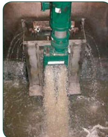
Muffin Monster in a pump station
